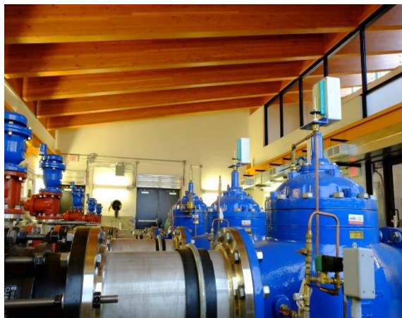
Valving inside the Energy Recovery Facility
