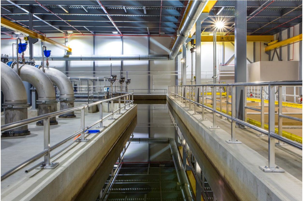
South Fork Water Treatment Plant – primary membrane raw water feed channel
