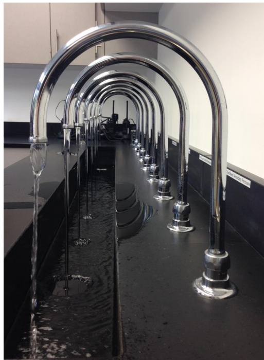
South Fork Water Treatment Plant – laboratory process water sample points
