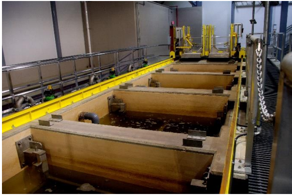
Raw (reject primary) water being filtered in secondary membranes
