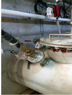
Primary and secondary membrane filtered water being treated at the chlorine injection point
