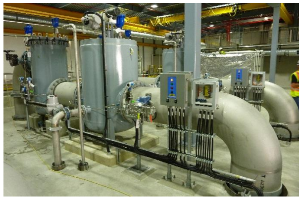
Raw water passes through coarse & fine screens
