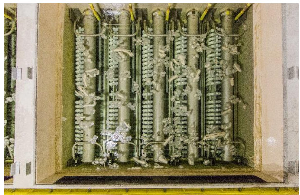
Raw water being filtered in primary membranes
