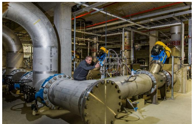
Raw water passes chemical injection points and mixing pumps
