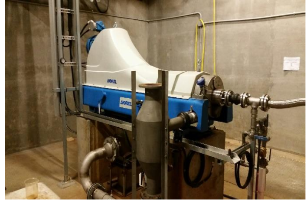
Reject raw water centrifuge
