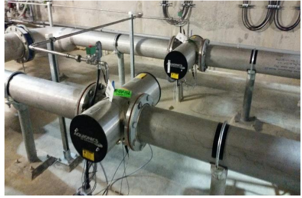
Secondary membranes raw water uv treatment
