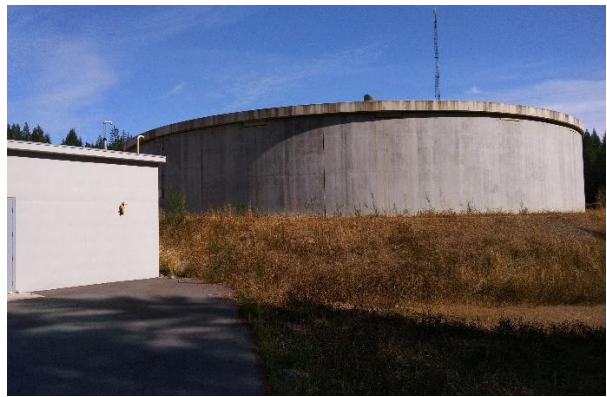
Treated potable water clearwell (storage tank)
